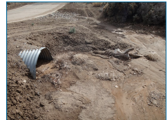
A culvert requiring maintenance in Douglas County. Photo courtesy of Douglas County staff.
